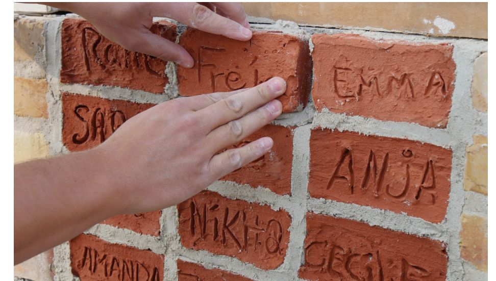
The bench is being built by masons assisted by the residents. Here the bricks with the names engraved are being placed as part of the bench.
