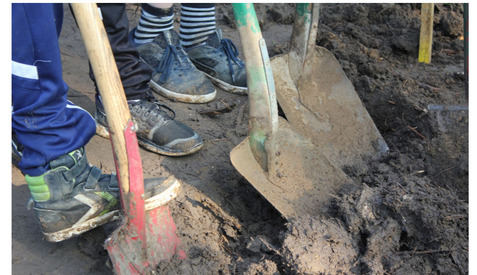
Pupils from the local school lay the foundation for The Brick Bench.
